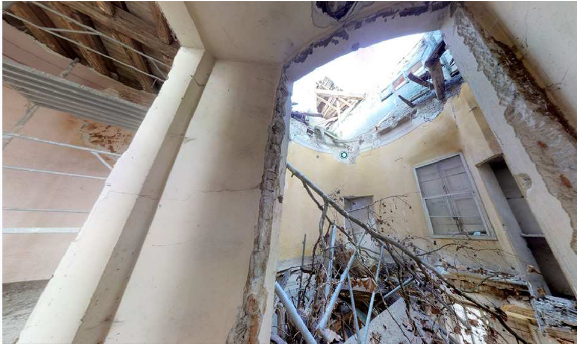
Fig. 3 – Portion of the first and second floor collapsed.
