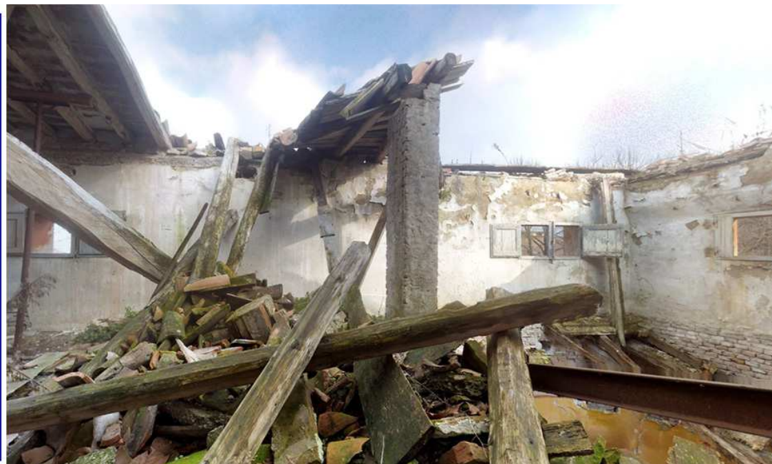
Fig. 4 – Portion of the roof collapsed.
